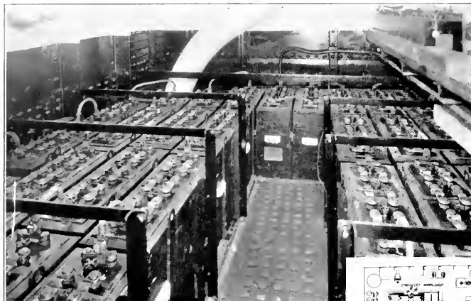
Above: the Exide storage battery installation in the special storage battery room.
